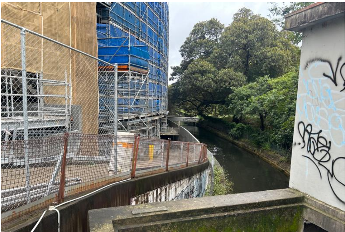
Figure 4: Rushcutters Bay stormwater canal which borders the east of the site, viewed facing north
